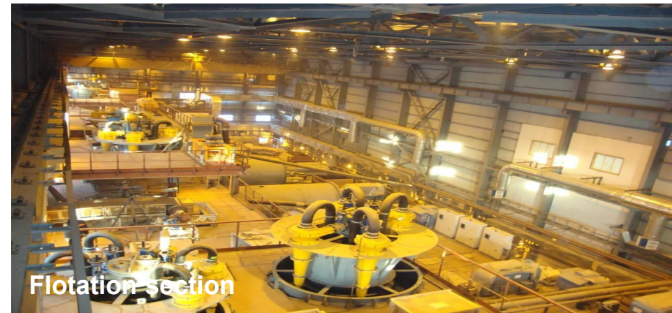
Flotation concentrator and ore preparation complex
